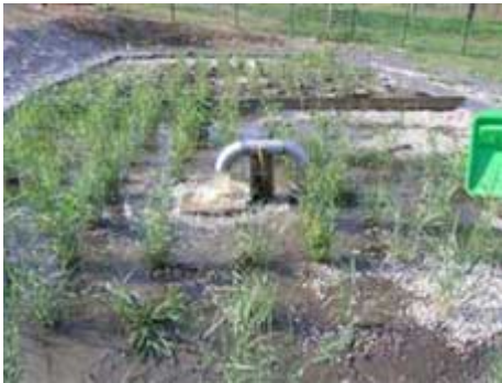
Feeding by "closed loop" type overflow via an underground system
