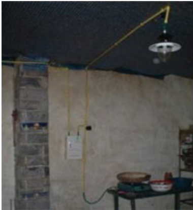
The lighting and stove of this house in China are powered by Biogaz
