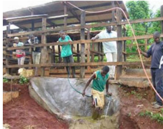
Filling a digester with diluted cow dung in another Biogas project in Africa. Photo Eric Florantin Tankeu
