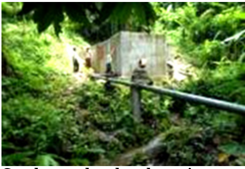
Catchment head and gravity water network in Laos (Photo UN Habitat)
