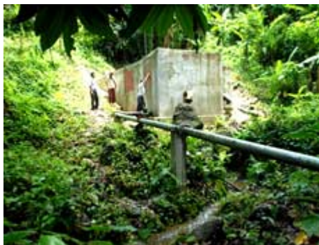
Spring catchment and connection to a network at Xieng Ngeun (Laos) (Photo un Habitat)
